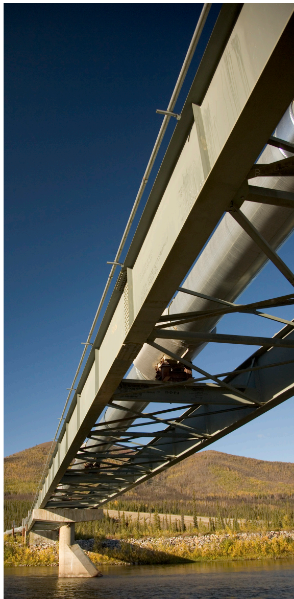
Trans-Alaska oil pipeline crossing on South Fork, Koyukuk River. S. Hillebrand, ADF&G.
