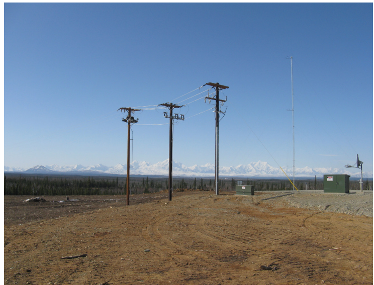
Utility lines under construction at Delta Junction, Alaska. ABR, used with permission.
