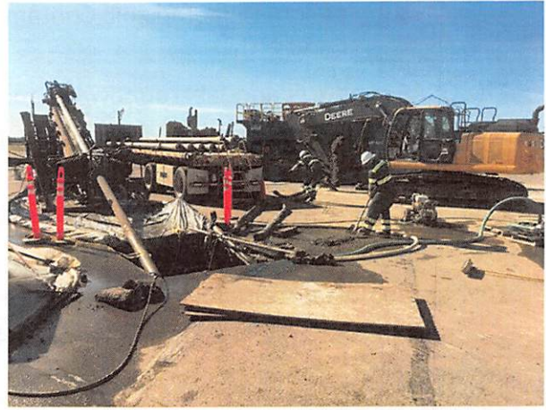
Advancement of a Horizontal Well at Galena FOL in summer 2017. The horizontal wells are approximately 1,000 ft. long and 45-75 ft. underground. Air will be injected into the wells to accelerate bioremediation of petroleum contamination in the soil and groundwater.
