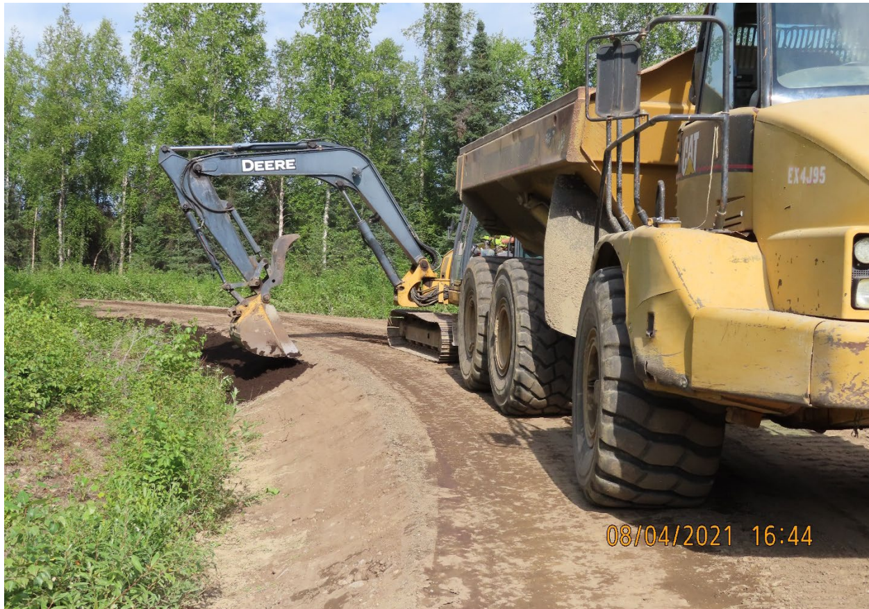
Figure 1.—Constructed road embankment section along Willer-Kash Road, with established ditches, fill slopes, and drainage transitions into existing adjacent vegetation.
