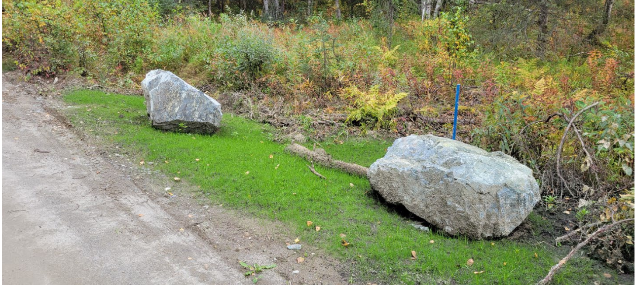
Figure 4.—Hydro-seeded and stabilized fill slopes at culvert install locations along Willer-Kash Road. Barrier rocks were installed to deter off-road parking and mitigate possible damage to the culvert structures due to vehicular traffic.
