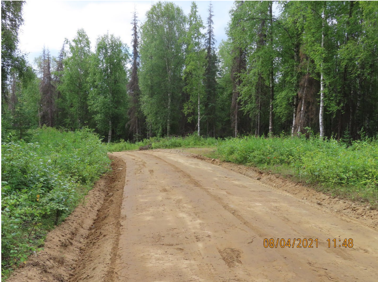
Figure 2.—Reconditioned road section with reestablished ditching for drainage purposes along Willer-Kash Road.
