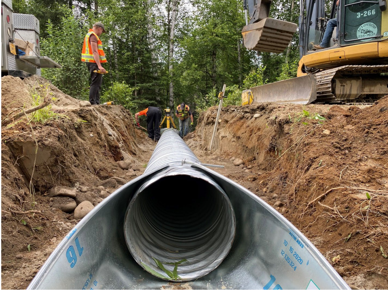
Figure 6.–Four culverts were installed to address road surface and surrounding area drainage.
