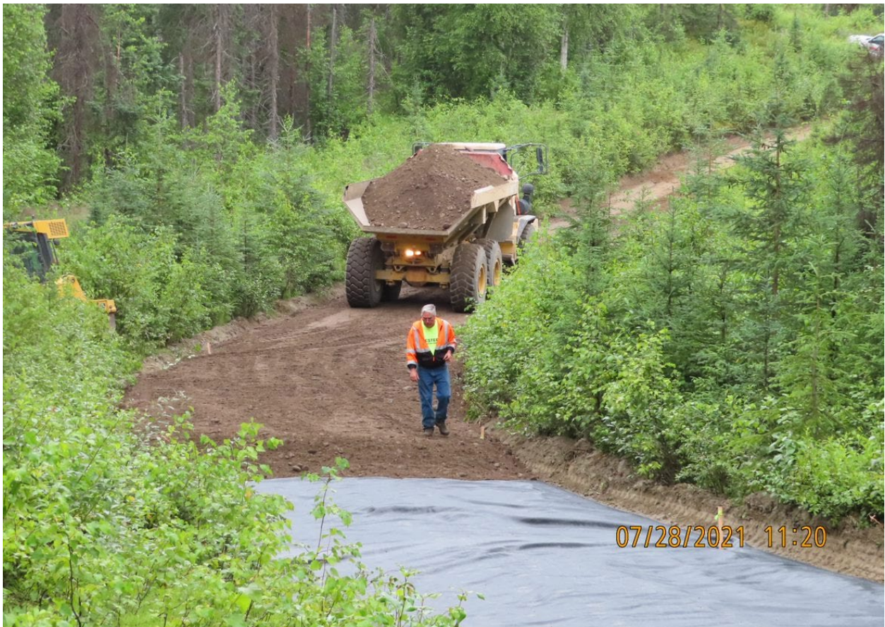
Figure 5.—Geotextile fabric was installed where surface fill was added to separate the two surfaces and improve long term stability of the road surface.
