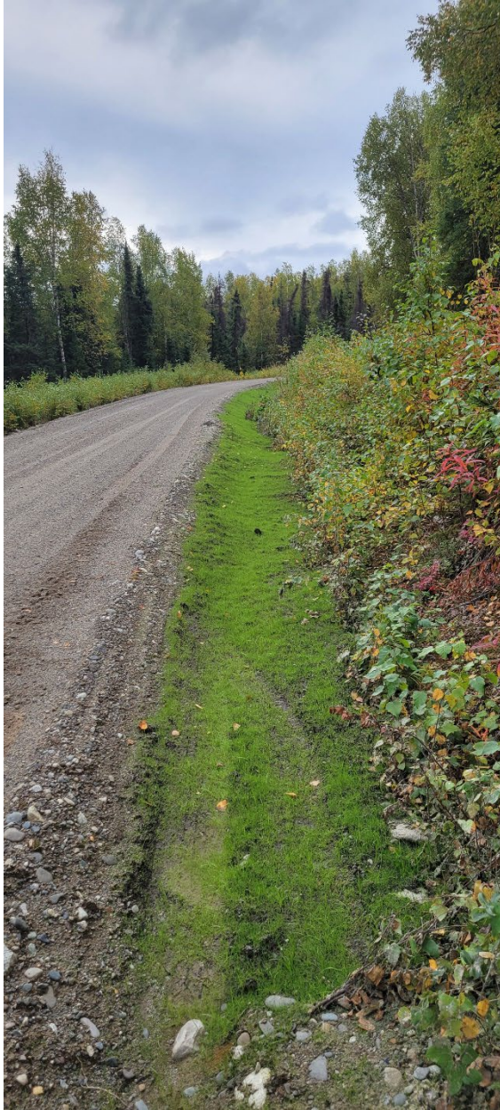
Figure 3.—Hydro-seeded and stabilized fill slopes on constructed road embankment sections along Willer-Kash Road.
