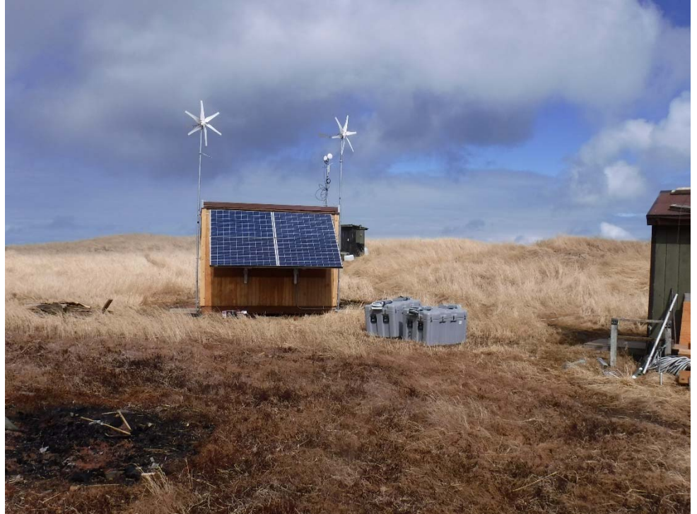
A new power shed was constructed to house Explore.org power and internet electronics in support of the live stream cameras.
