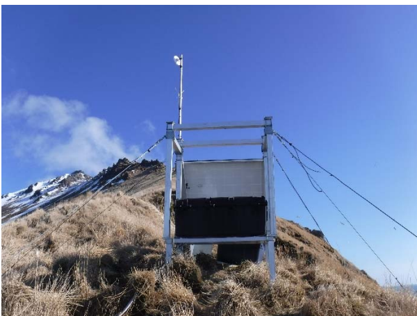
West Main Beach repeater station.
