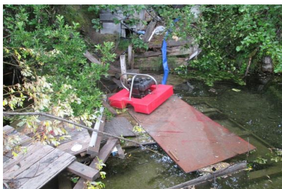
Figure 2.–Water intake on creek near camp.
