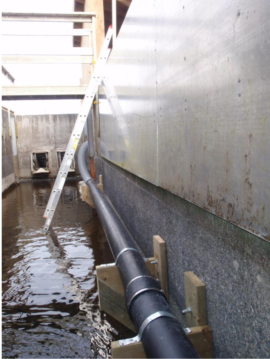
Figure 7.—Existing smolt pipe assembly situated in the adult counting structure.
