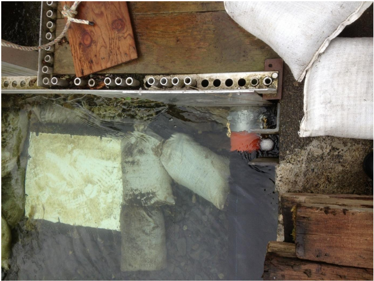
Figure 6.–Smolt pipe connection through the adult counting structure.
