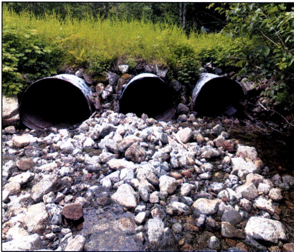
Figure 3.—Substrate impounded upstream of culvert inlets at waypoint 435.
