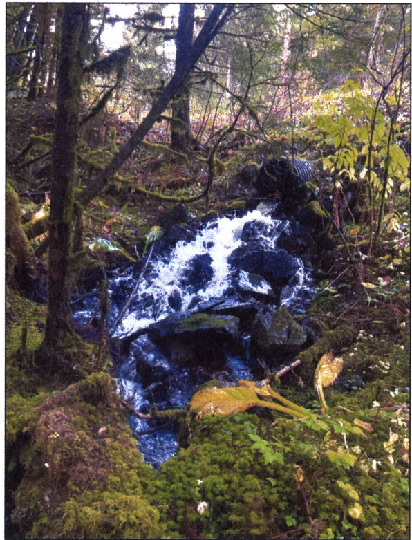
Figure 3.—Perched culvert outlet at waypoint 1034.
