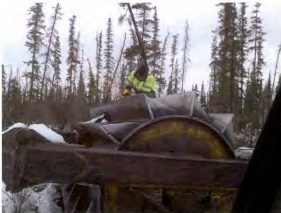
Figure B-10. Grinding of the chopper fins is critical to getting good ground penetration and chopping of tree trunks.
