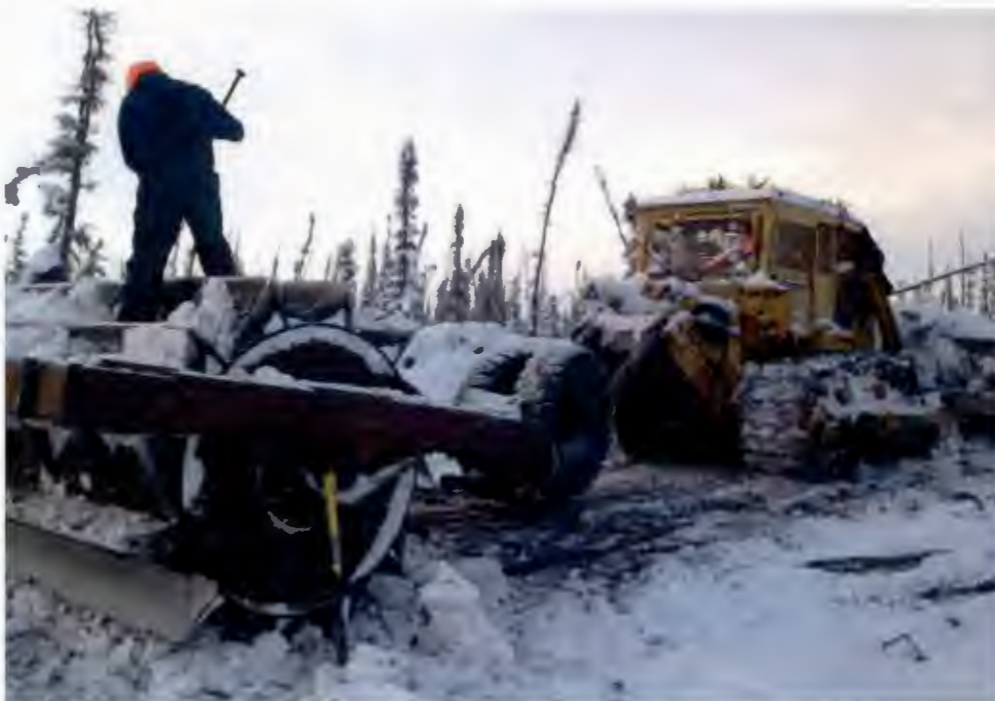
Figure B6. Cleaning snow compaction on roller chopper after snow reaches 24". Snow compaction reduces effectiveness of the roller chopper for ground penetration and cutting tree trunks.
