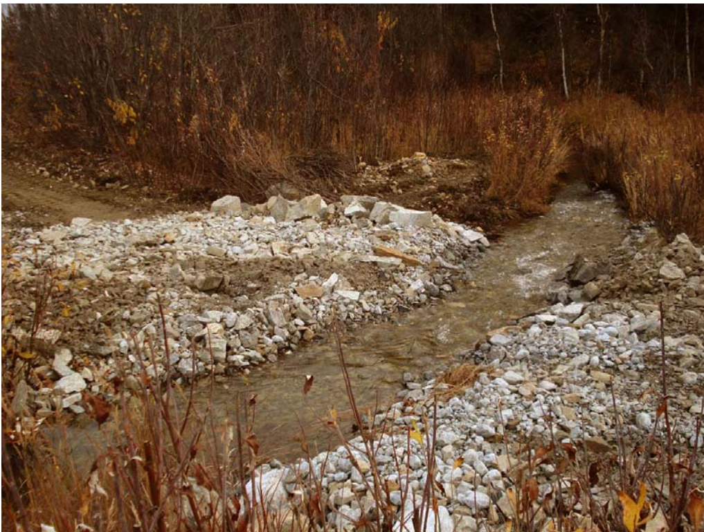
Figure 2. Last Chance Creek after channel excavation and backfill with granite (photo courtesy of FGMI, fall 2008).
