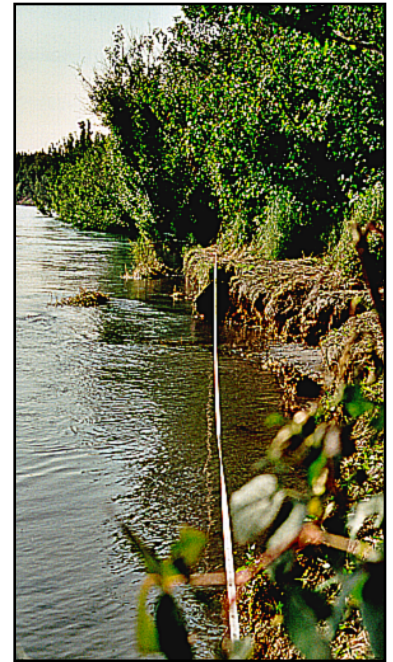
Significant bank loss.
