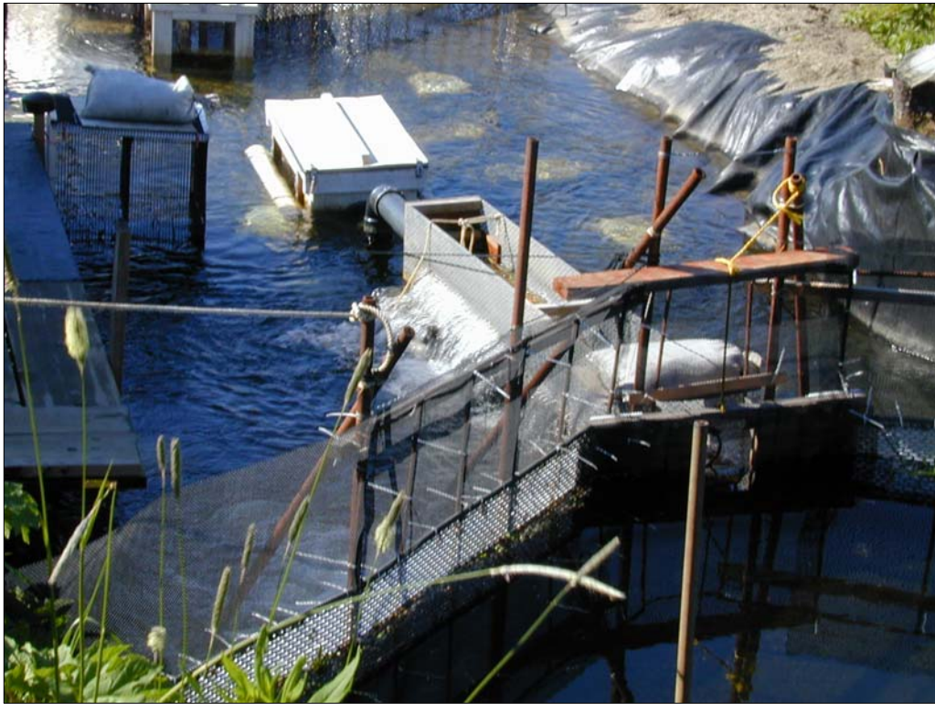
Figure 19. —Spill trap weir combination. Note bank stabilizing efforts, and the use of perforated metal panels and plastic cable ties.
