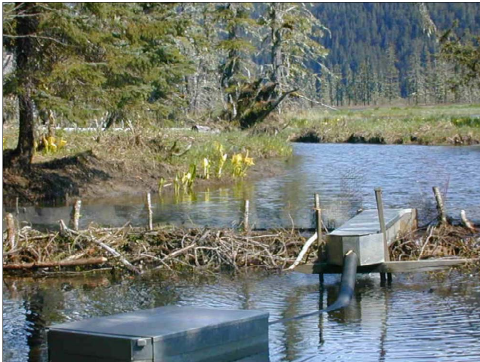
Figure 18. —A spill trap is installed in a beaver dam taking advantage of an 8-in difference in water level. Numerous small trickles are blocked by a fence of mesh on the inside slope of the dam. The mesh fence is also a preparation for higher water levels. Note floating aluminum live box with solid lid.
