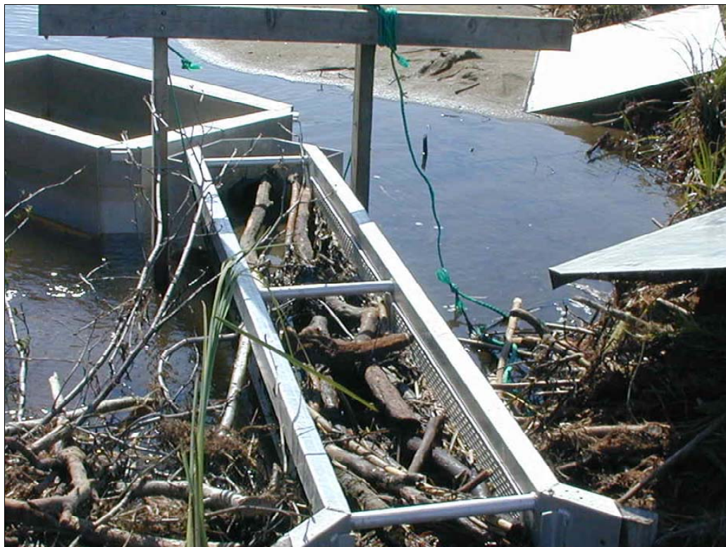
Figure 22. —This spill trap was plugged by a busy beaver. This photo illustrates one reason that daily inspections are needed even when fish numbers are low.
