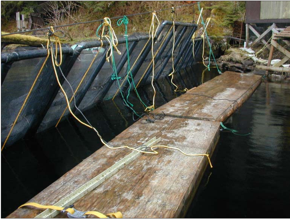
Figure 17. —The smolt weir panels at Hugh Smith Lake are constructed of four-inch ABS plastic pipe and covered with ¼ inch mesh Vexar®. The panels rest against the lake bottom and are supported by a cable at the top.
