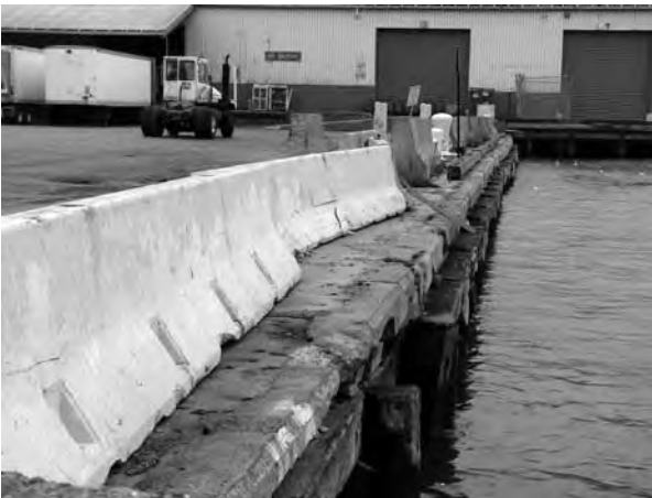
This row of concrete bulwarks provides a good rat travel route. Defensive stations could be spaced along the seaward side.
