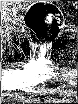
Above: Culvert acting as fish barrier
